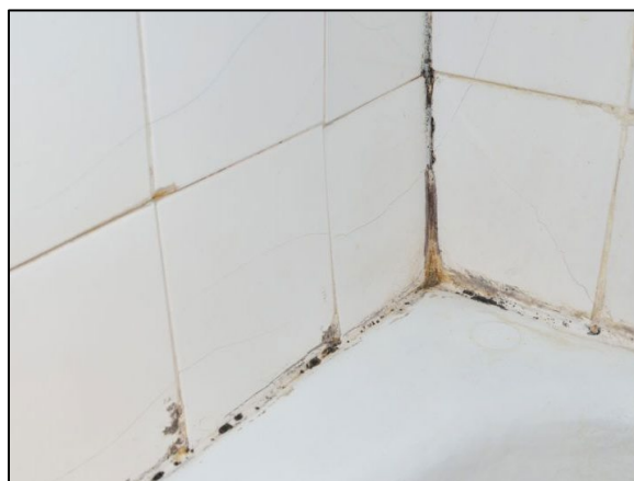
Mildew found on bathroom grout
