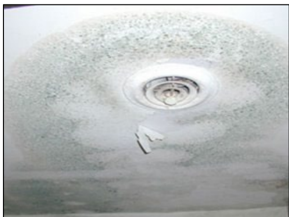
Mold surrounding air conditioning vent
