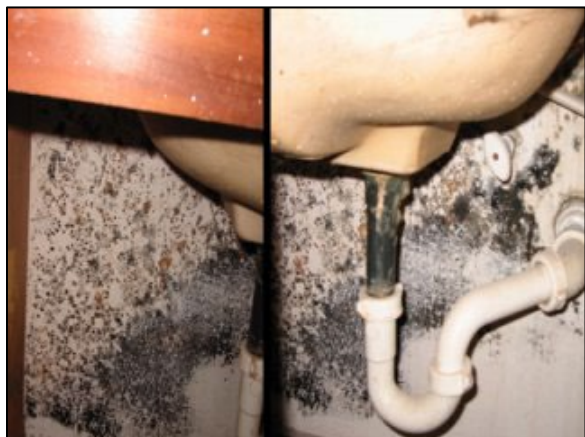
Mold on drywall under leaky sink
